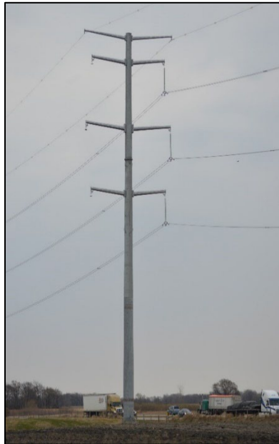
Figure 2-1 Existing 345 kV Structures on Eastern Segment
