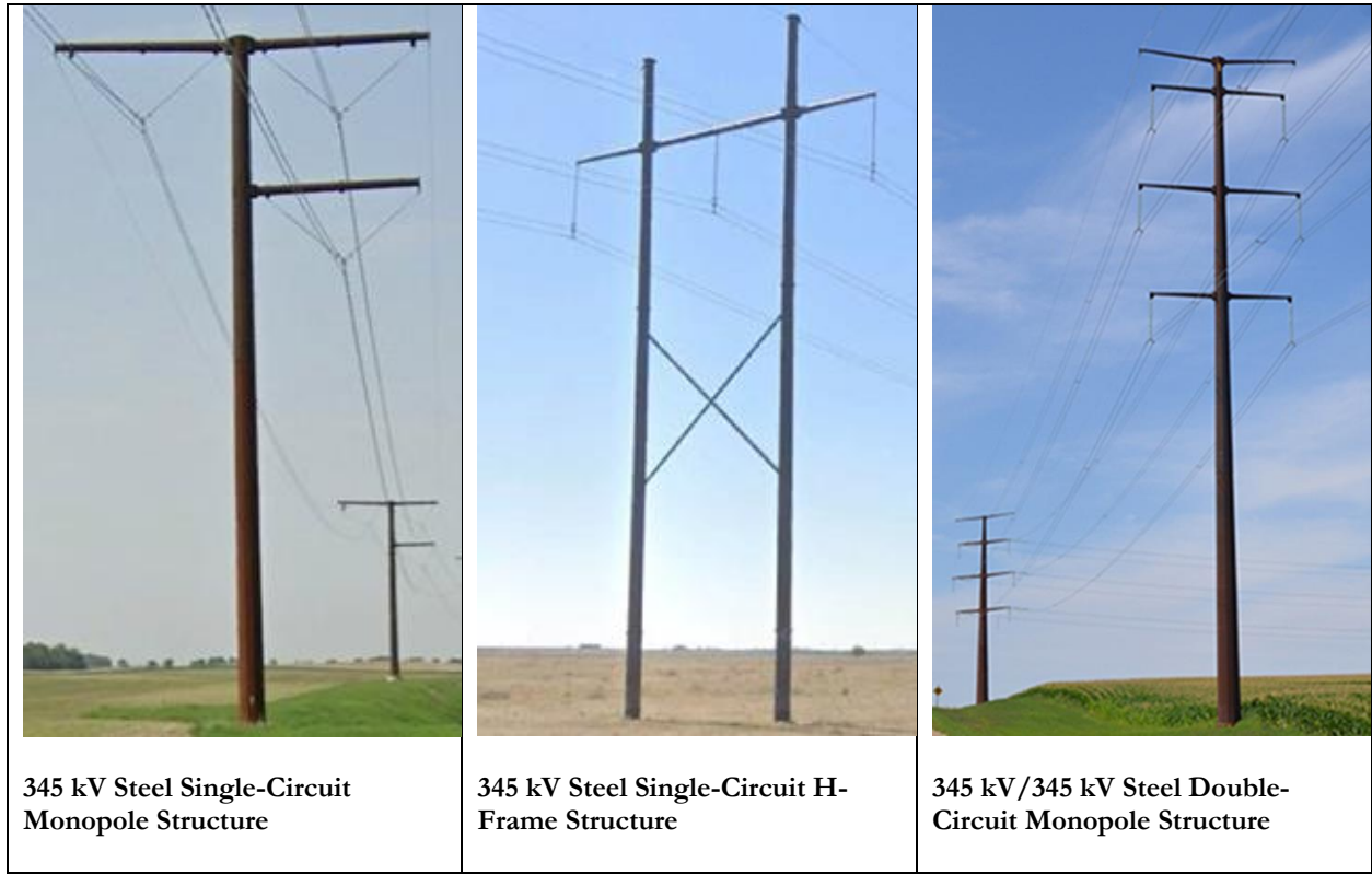
Figure 2.5-2 Typical 345 kV Structures
